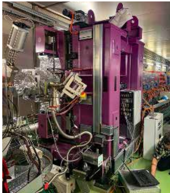
Figure 14. XAIRA's in-vacuum undulator installed in the Storage Ring.
